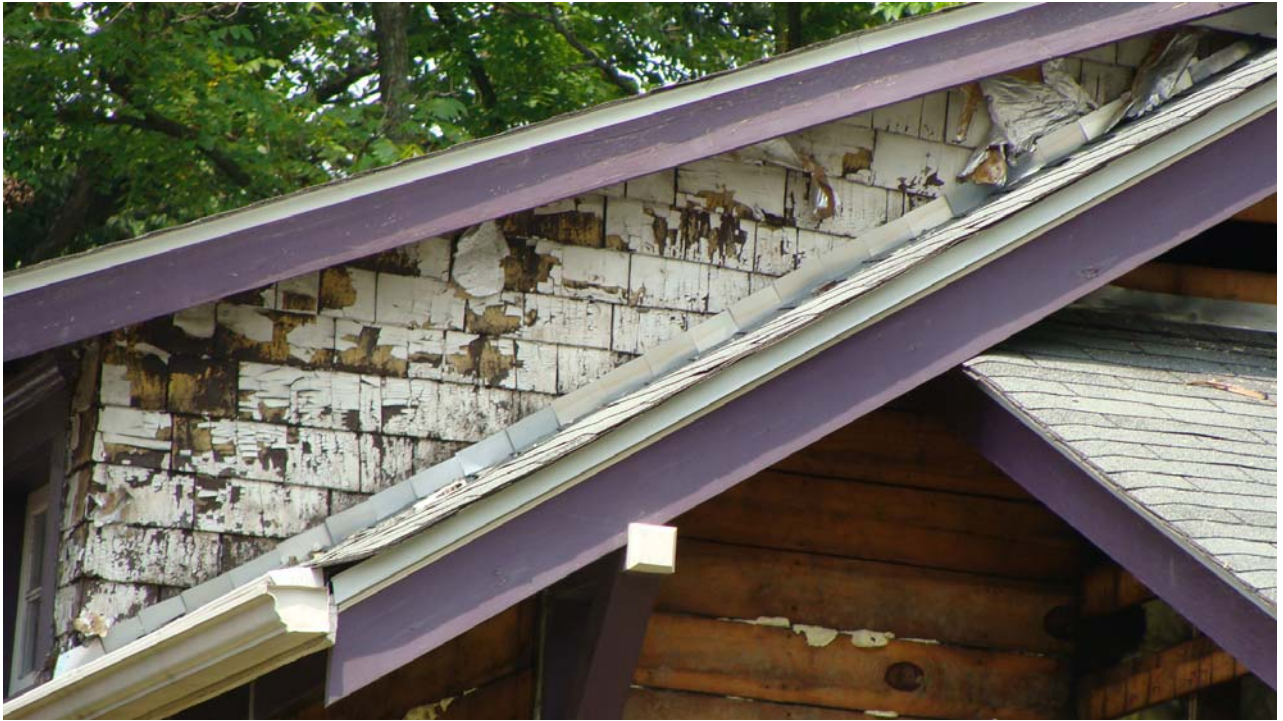
Above: View of wood shingles in one of the two dormers. This detail was revealed when the aluminum siding was removed.
