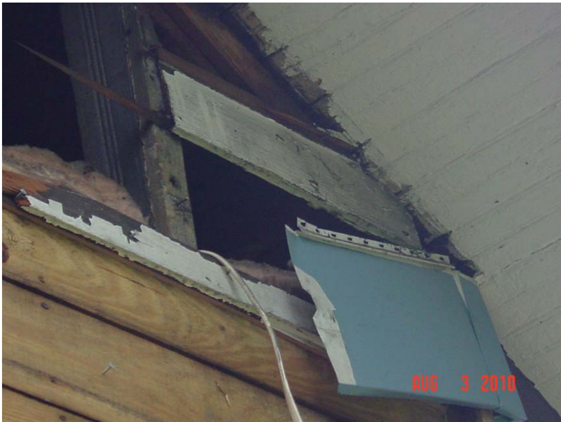
Below: View of one piece of wood siding that was left on the house. This piece is located on the rear of the house.
