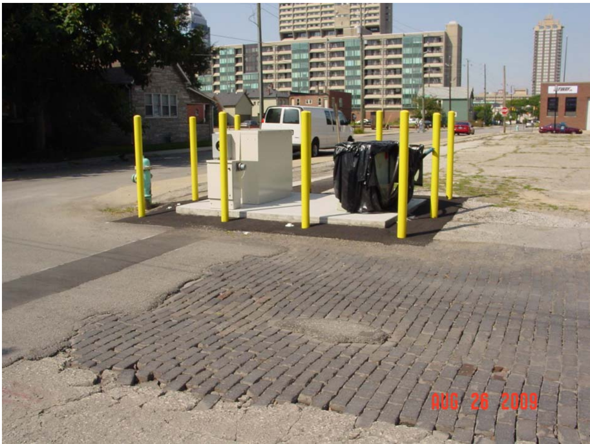
Installation before bollards were altered.
