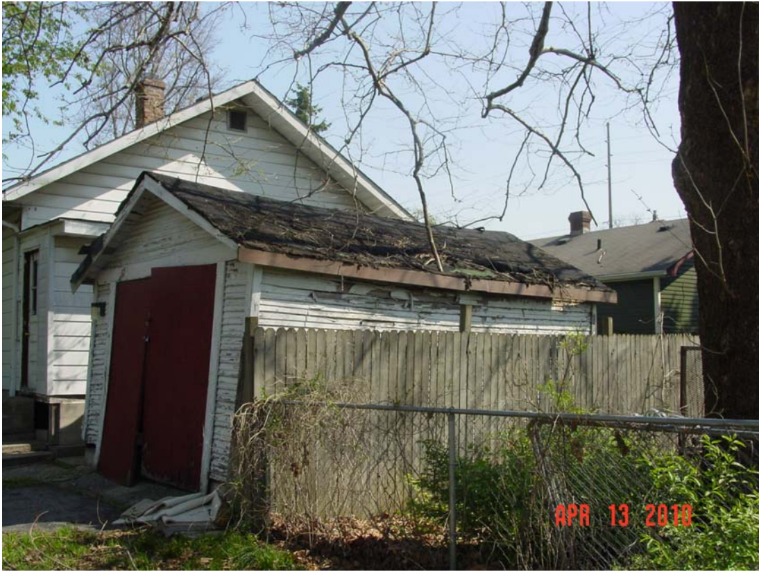
South side of garage; note holes in roof
