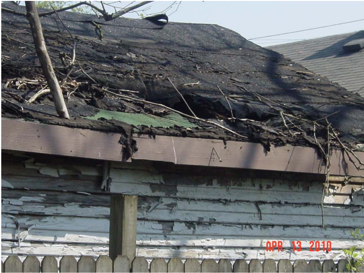
Detail of failing roof
