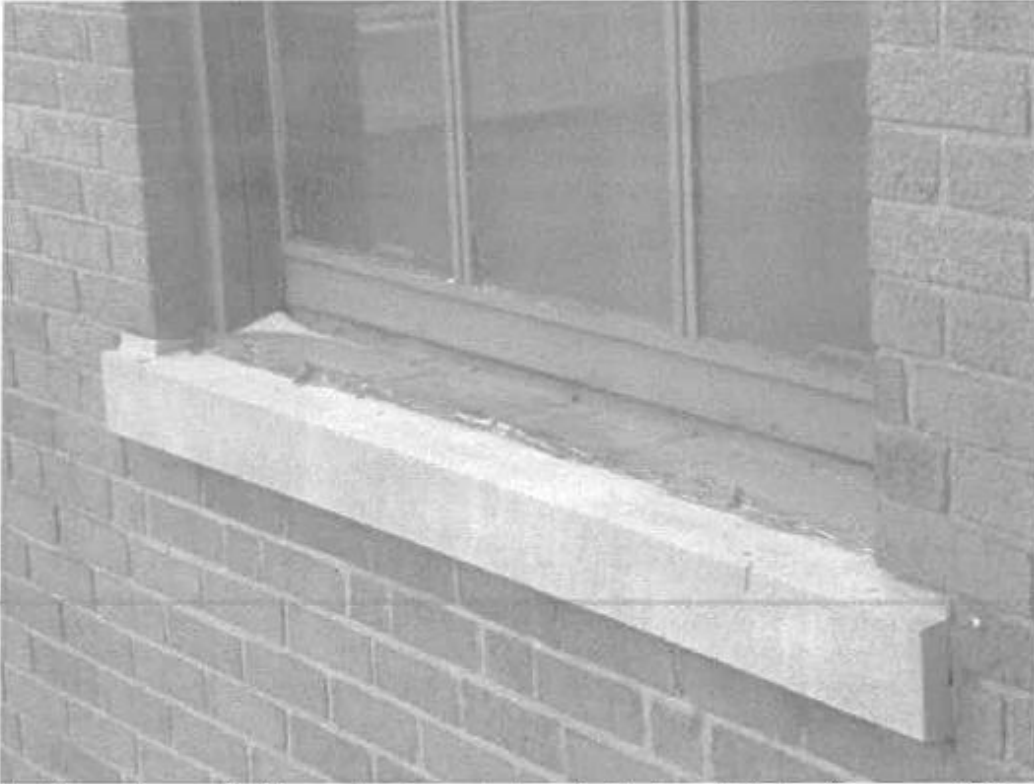
Peeling paint and failing sealant at exterior of window. Exterior faces are difficult to reach due to height and location above sidewalks.
