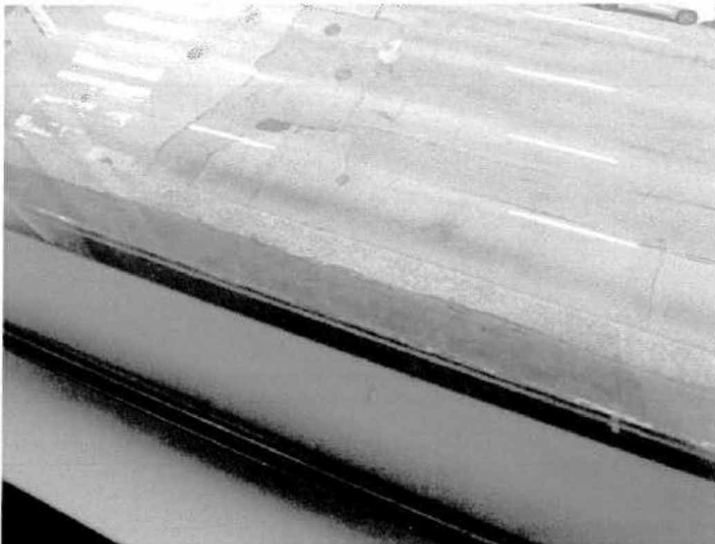
Corrosion at exterior sill
