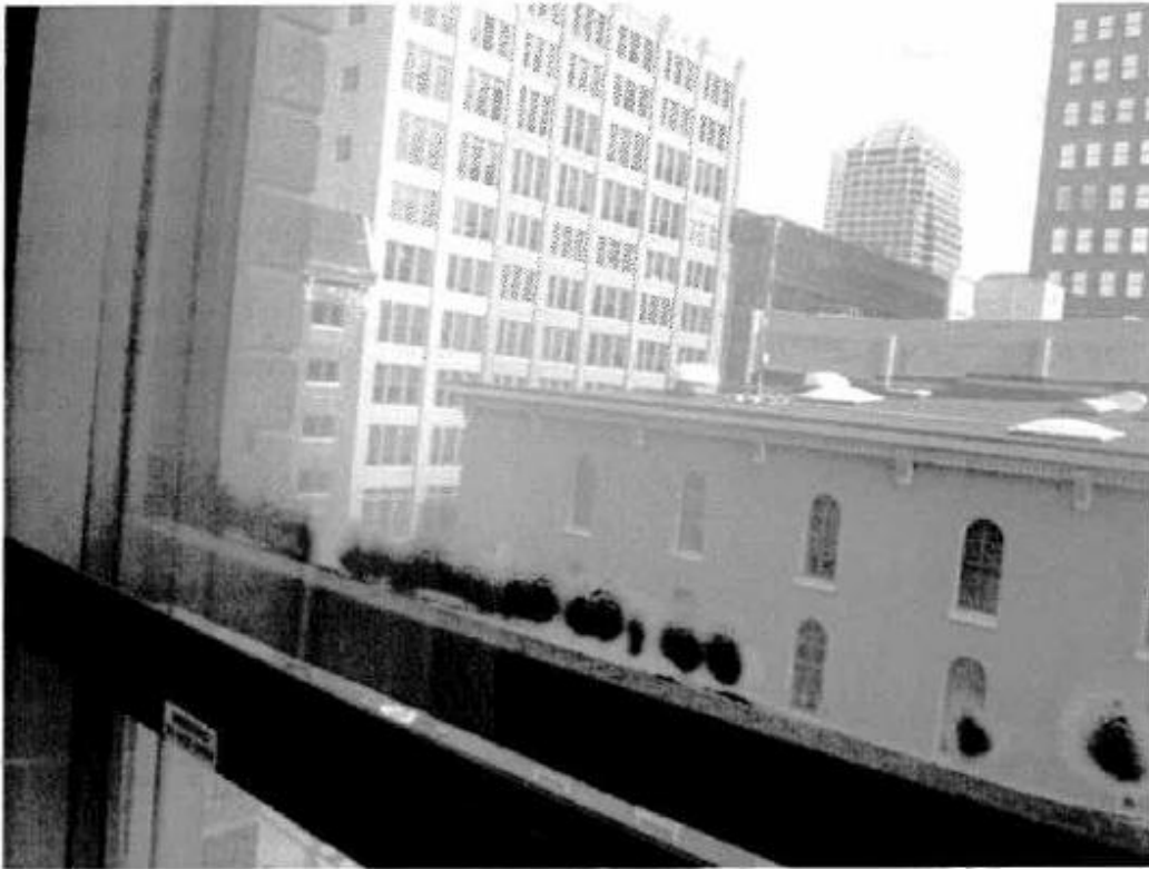
Mold growth between interior storm and window.
