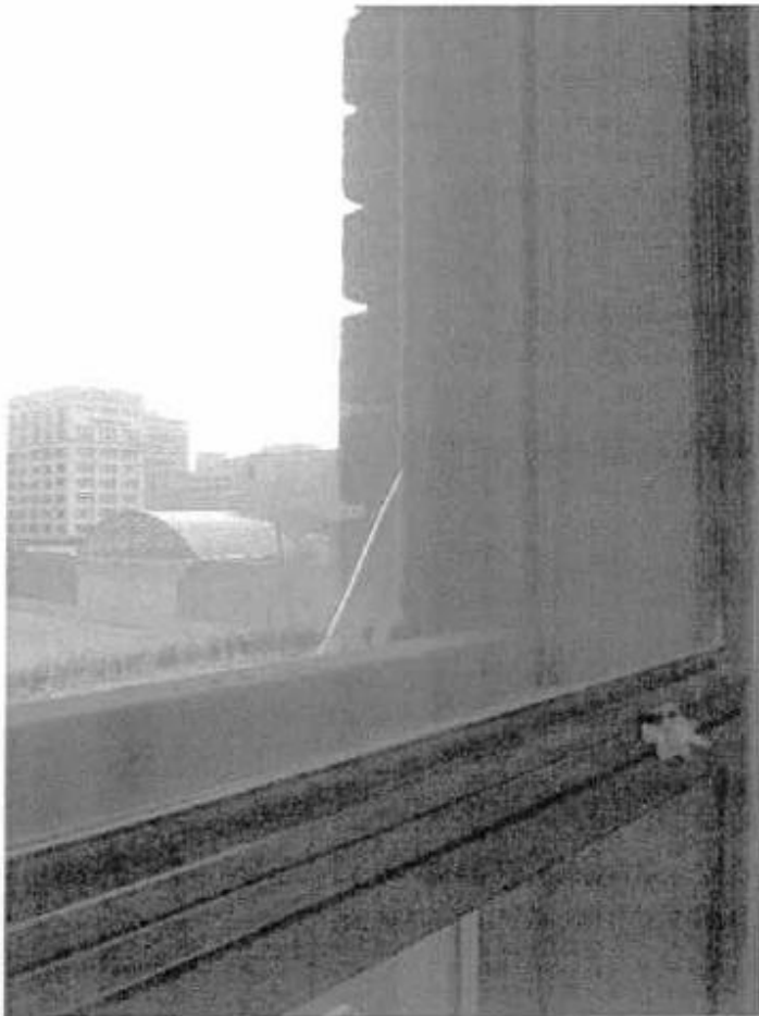
Broken Glass – Corroded steel is expanding, putting pressure on the panes of glass which then fracture.
