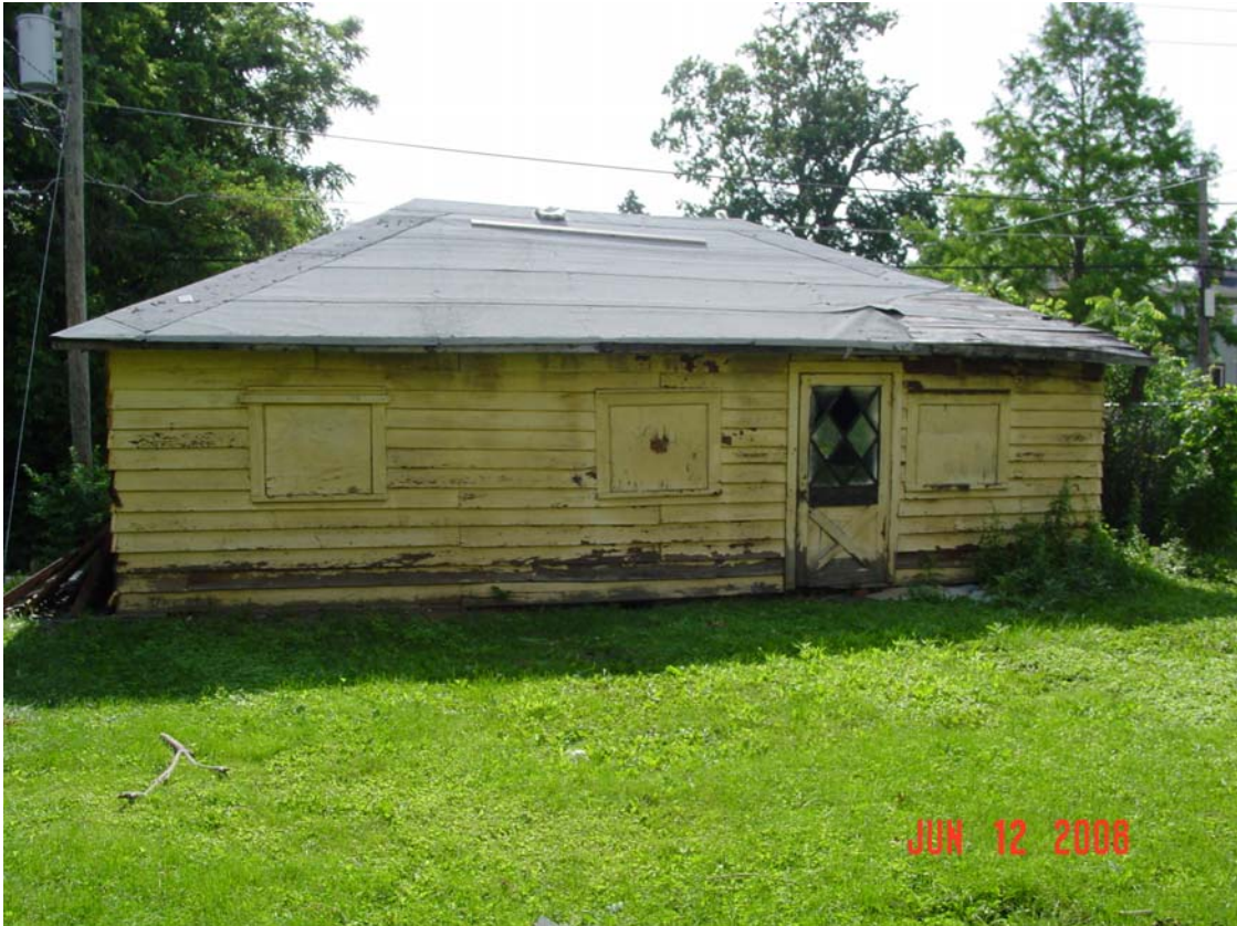
West elevation of garage facing back of building (wall is currently bowed out)
