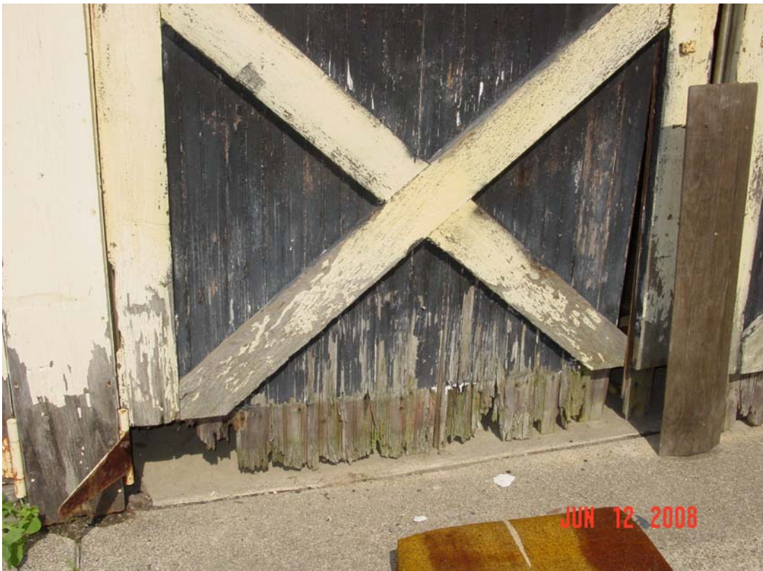
Bottom of one of the three garage doors
