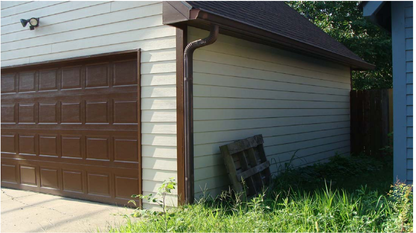
View looking at the northwest corner of the garage seen from the alley
