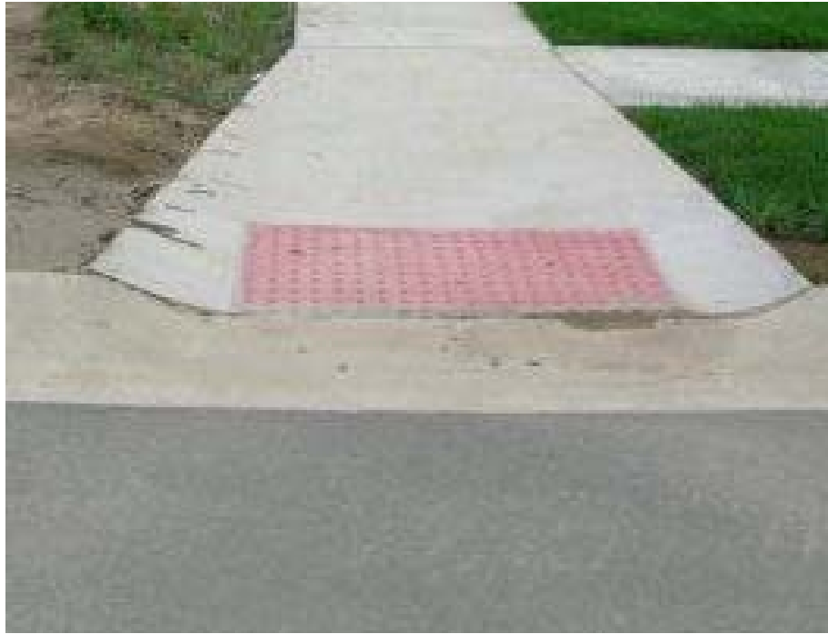
Above: Typical ADA-compliant sidewalk ramp Below: Existing sidewalk ramp at southwest corner of Delaware and 16th
