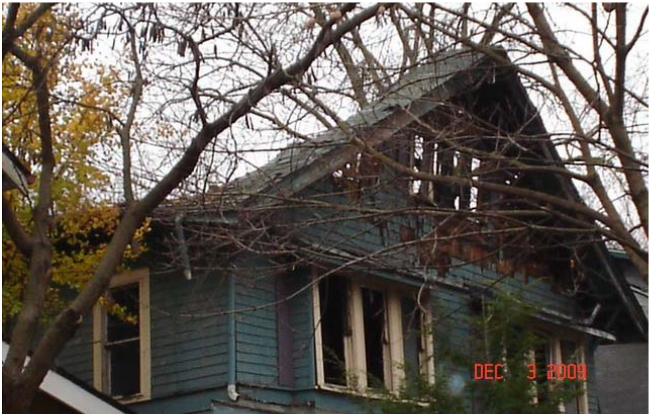
December 2009 – front gable required emergency demolition
