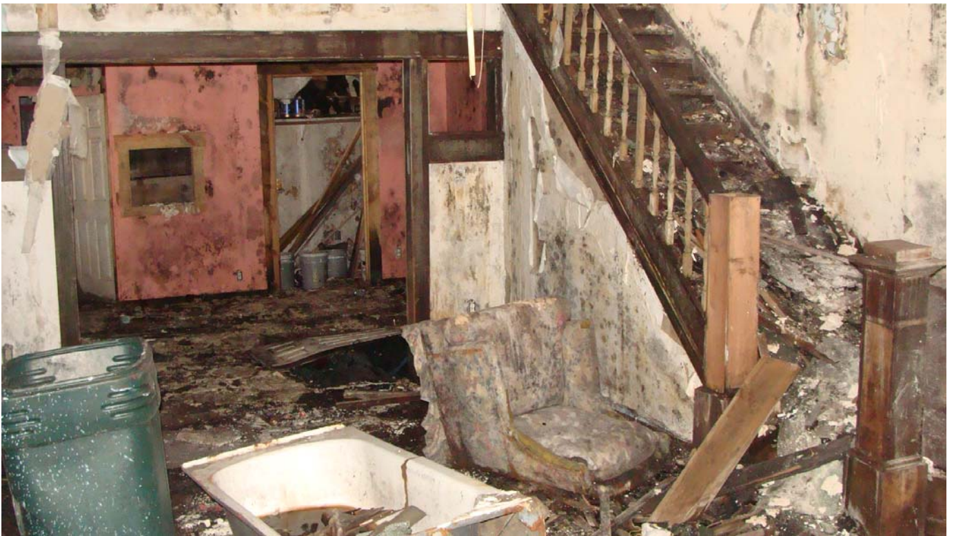
Interior at first floor- Black mold covers the area
