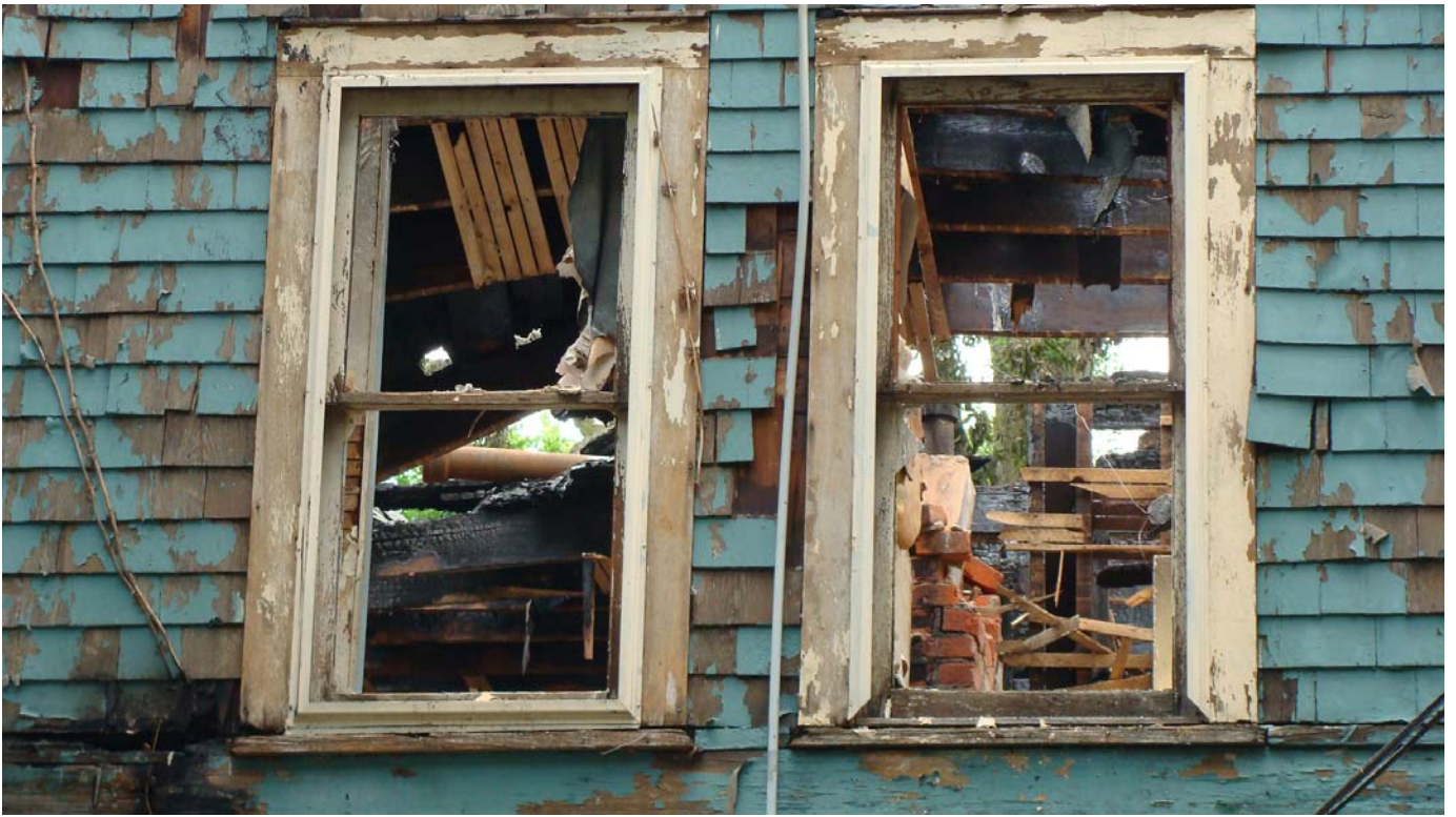
Close up of second floor rear windows- windows were blown out
