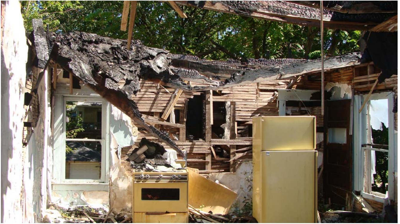
Interior at second floor- No roof remains
