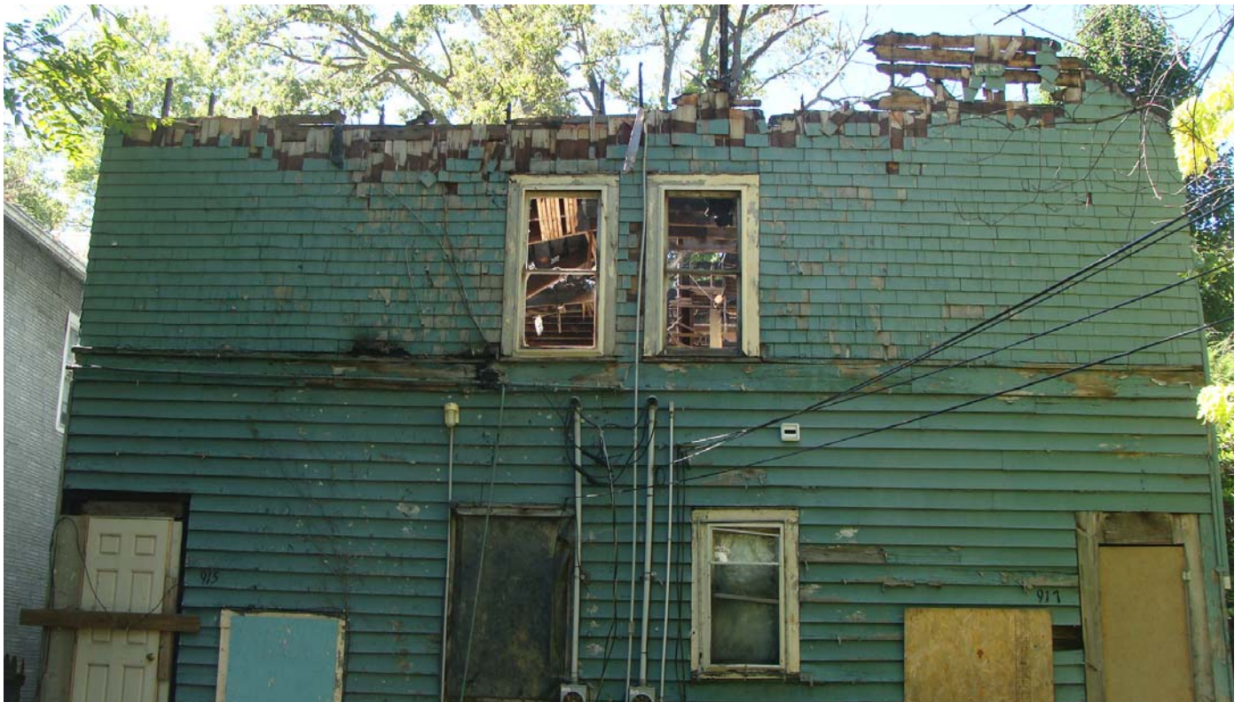
Rear of building- No roof exists
