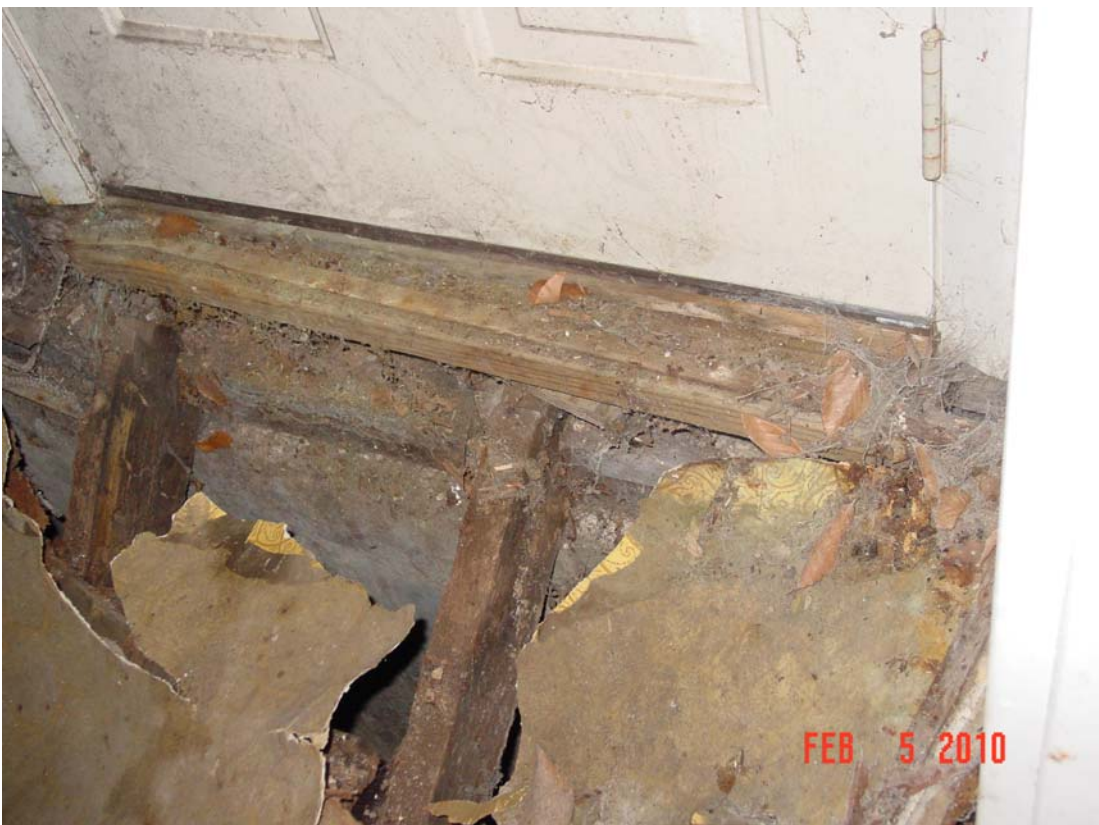
Partial collapse of floor near exterior door
