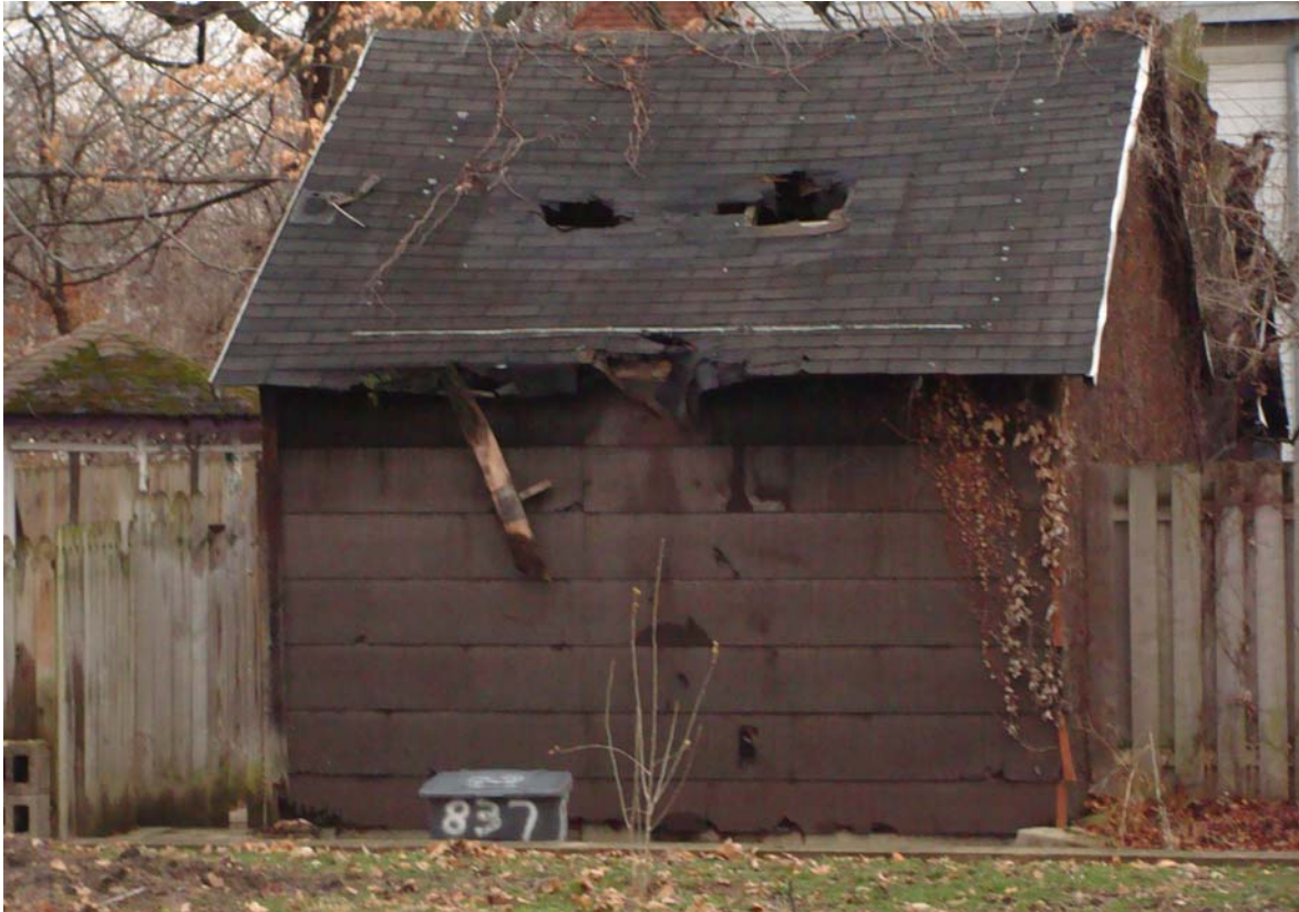
Photo showing existing condition of rear historic garage (taken by staff from neighbor's yard)
