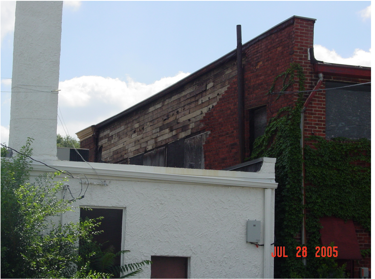
Veneer failure evident in 2005
