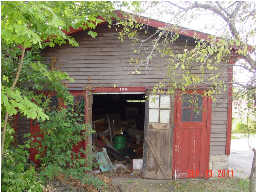
Above: View of north side of garage as seen from 19 th Street. Notice lean at right.
