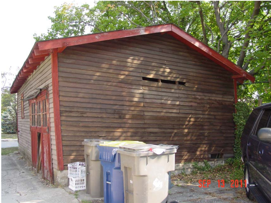
Above: View of south elevation of garage. Notice lean in wall at alley side.
