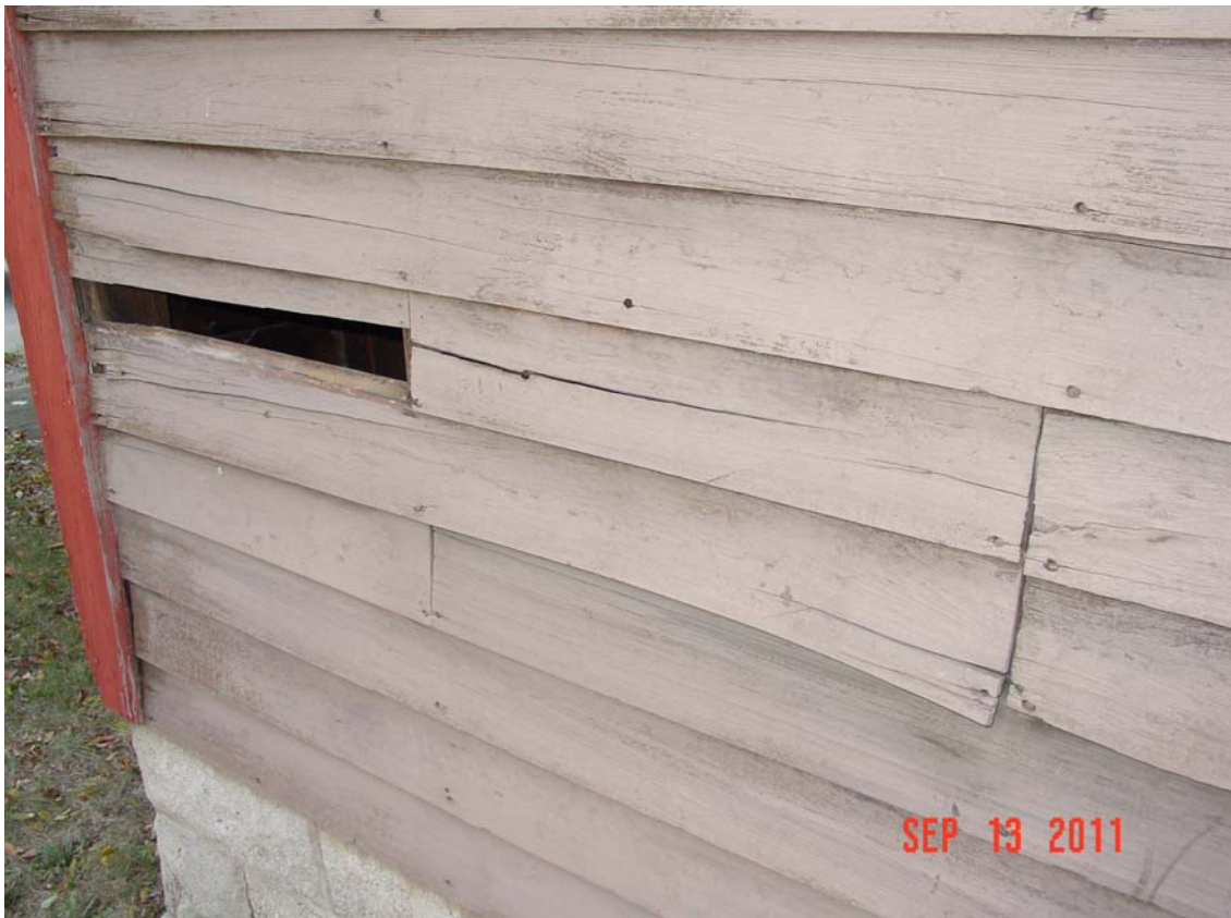
Below: Siding is dry, curling and brittle with many splits. Siding is not the original siding on the structure.
