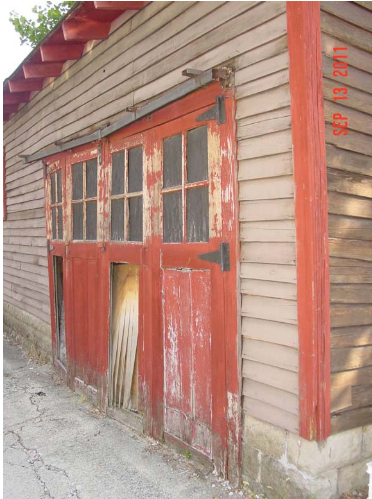
Above: View of doors on alley side. Doors appear to be historic, but are in poor condition.
