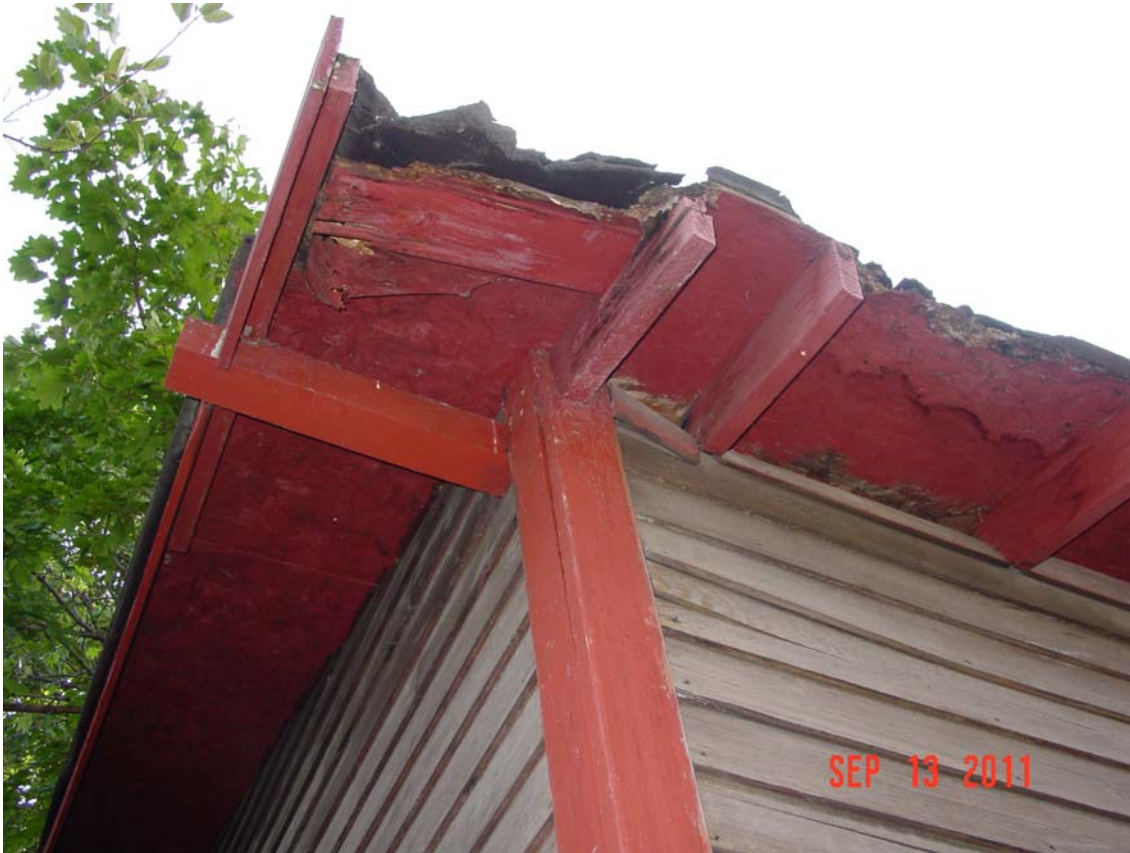
Above: View of non-original plywood at eaves and deterioration of eave material.
