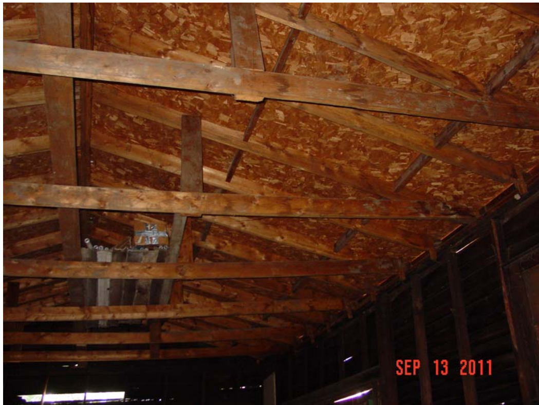
Below: View of replaced roof structure from the interior of the garage. Roof sheathing and trusses have been replaced
